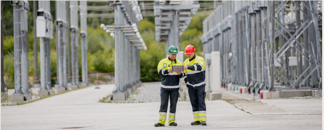
Consistent instructions and procedures for electrical safety are crucial at Statnett. Photo: Terje Borud/Statnett.
